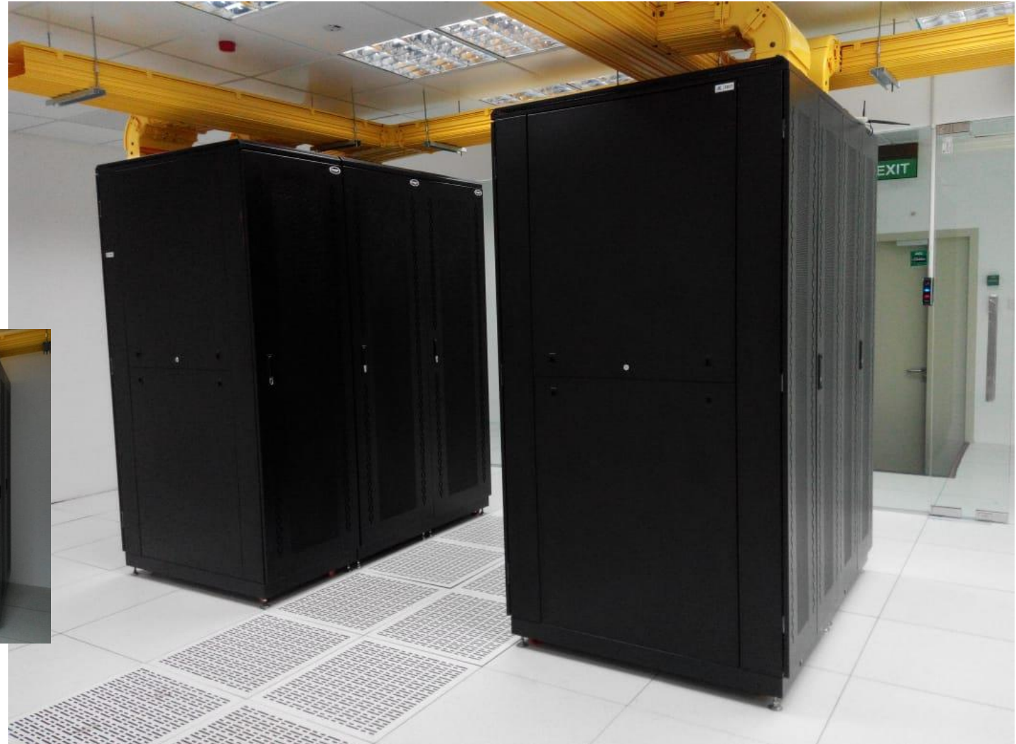
Ruang server, storage dan access system
