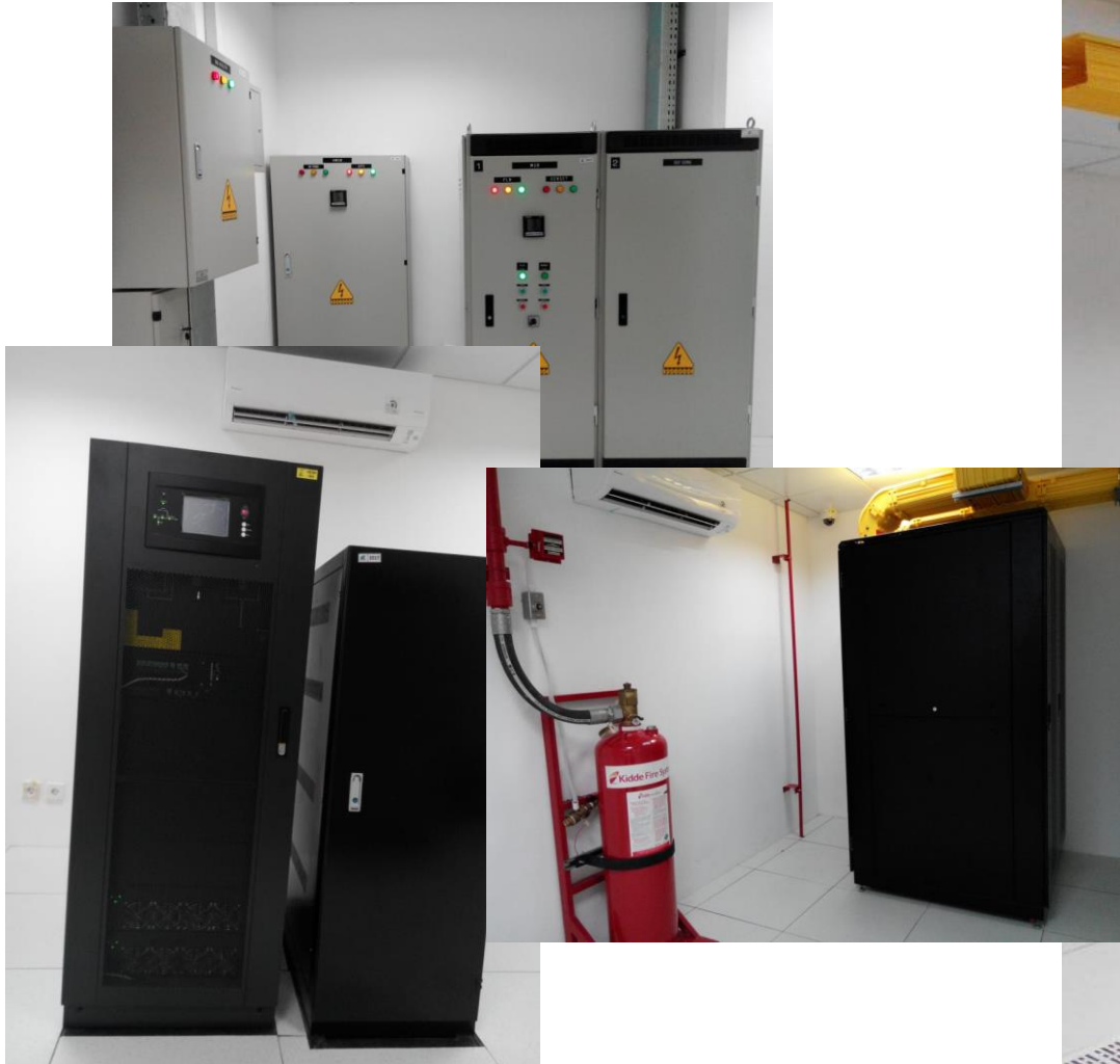
Ruang panel, fire suppression system, access control dan UPS
